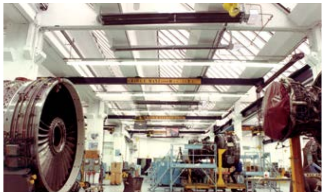
⚡ Aircraft hangars (top photo) and an assembly line (above photo) use tube-style radiant to warm objects and maintain indoor air comfort for employees.
